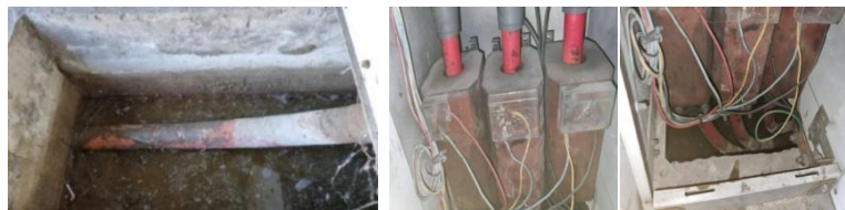
Figure 5. Flooded Cubicle Ducting and Burnt, Physically Cracked CT on the PLN-Side Cubicle
