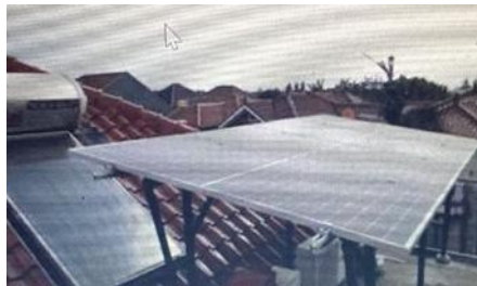
Figure 3. Photovoltaic Power System at PT. Icon Plus Pekanbaru
