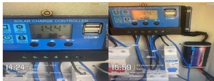
Figure 6. Battery Charging Results Observed from the Solar Charge Controller
