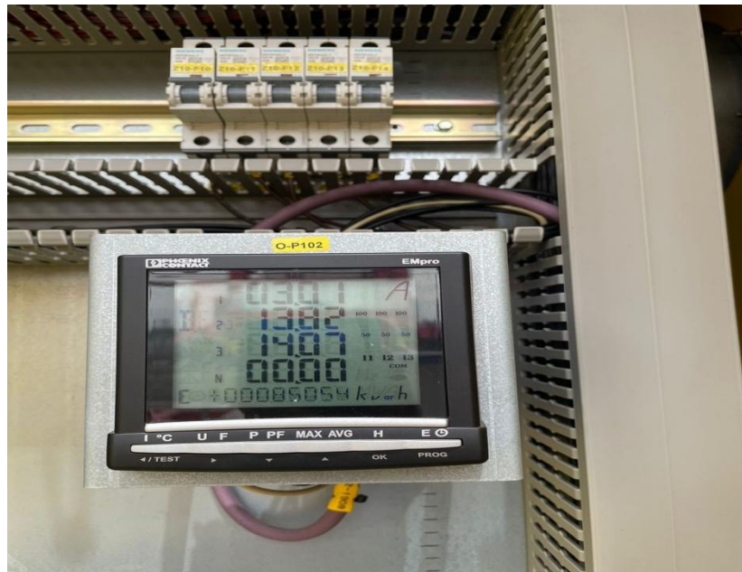
Image 1 Energy Measuring Instrument and Electrical Parameters in Dry Transformers
