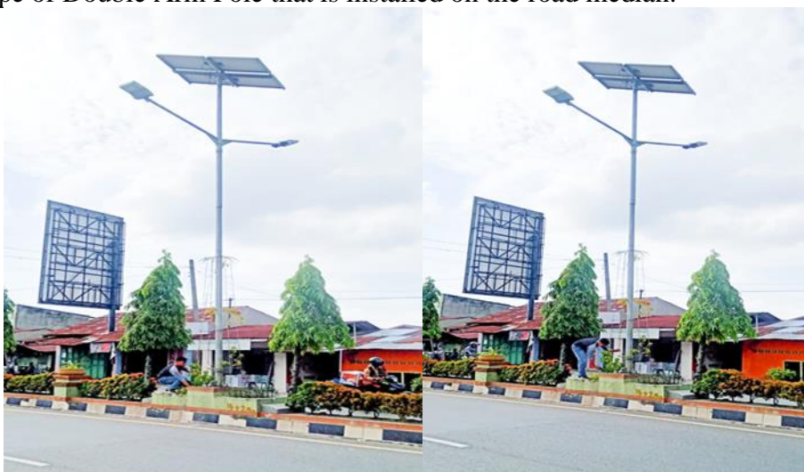
Figure 7. Type of Double Arm Pole in the Road Median
